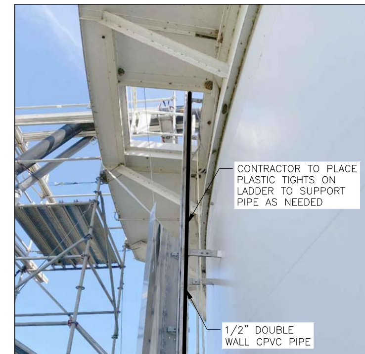
7 APPROXIMATE PIPE LOCATION
