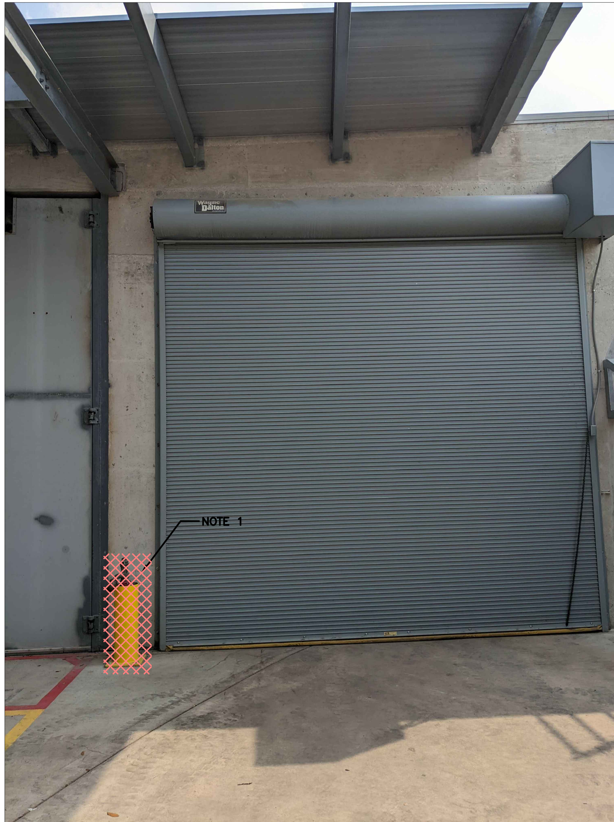
HYDRANT DEMO EXISTING CONDITIONS AT EAST OVERHEAD DOOR SCALE: NTS
