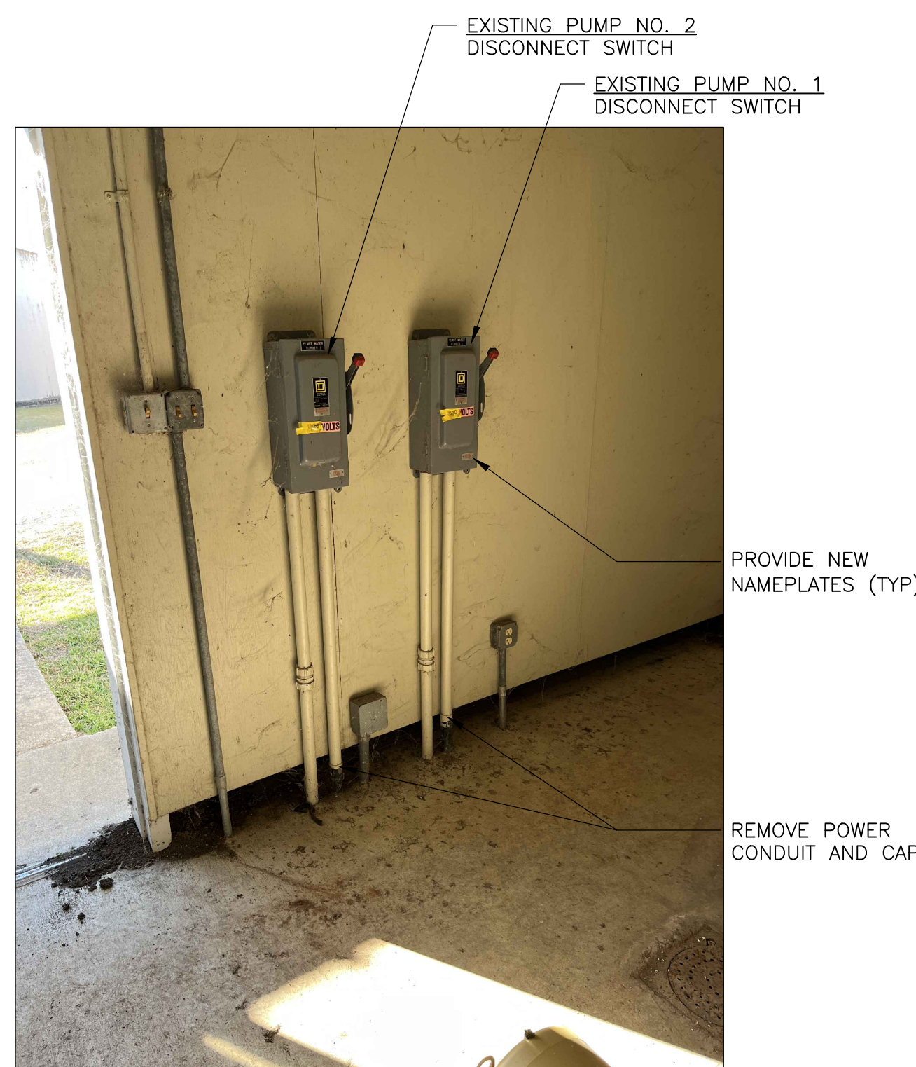
EXISTING DISCONNECT SWITCHES PHOTO 1 SCALE
